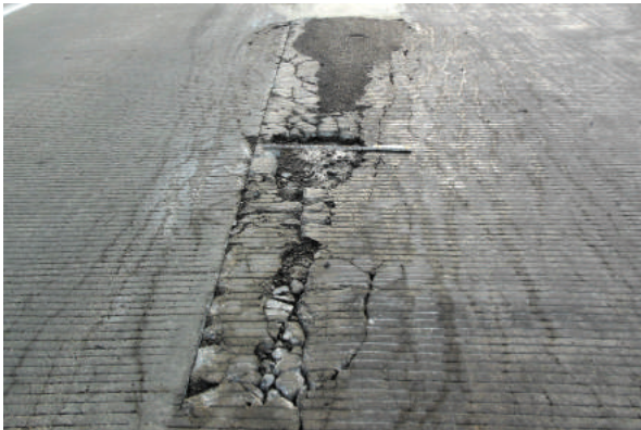
Concrete slab spalling.
