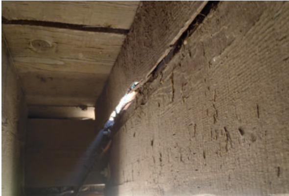
Cracked timber stringers.
